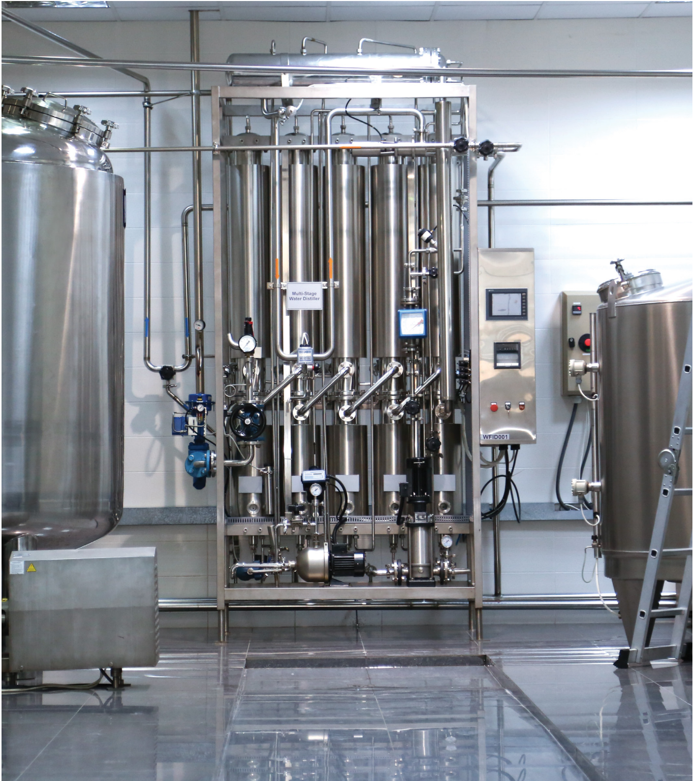
MULTI-STAGE WATER DISTILLER, LIQVOR PHARMACEUTICAL COMPANY
