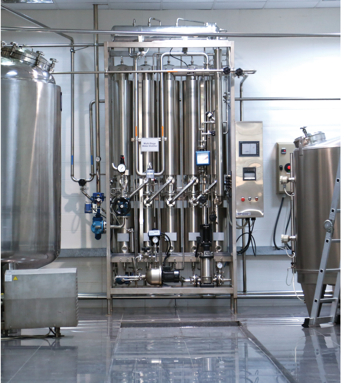
MULTI-STAGE WATER DISTILLER, LIQVOR PHARMACEUTICAL COMPANY
